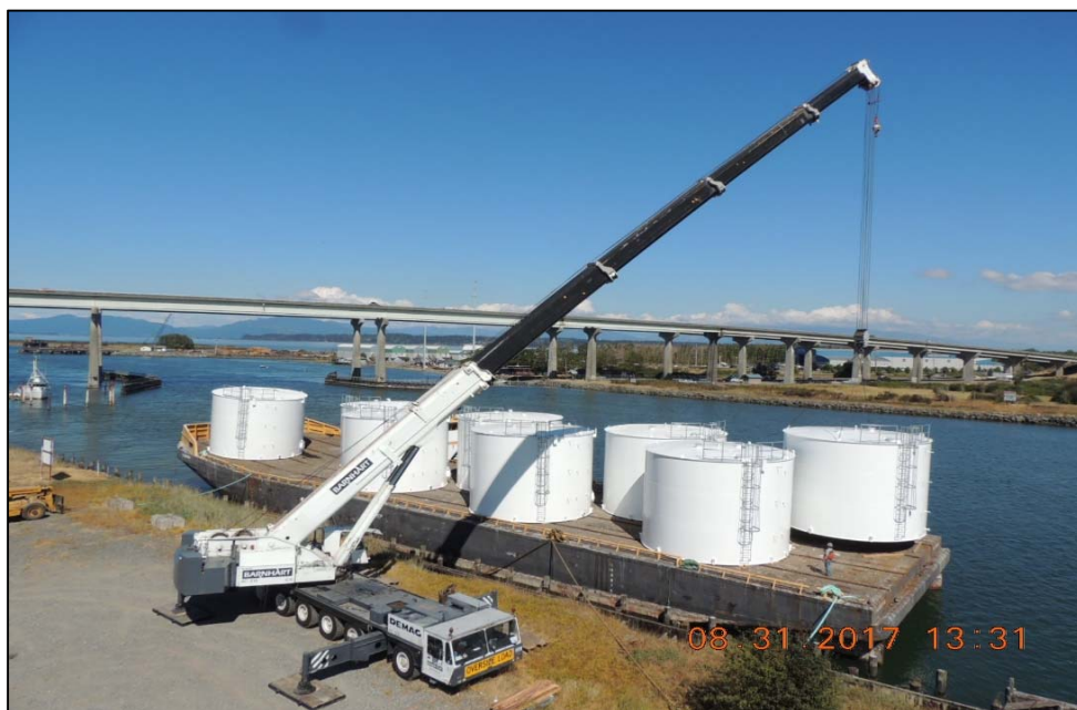
Kipnuk Bulk Fuel Tanks
