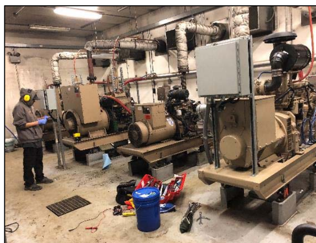
Hughes powerhouse operator during May 2018 electrical emergency
